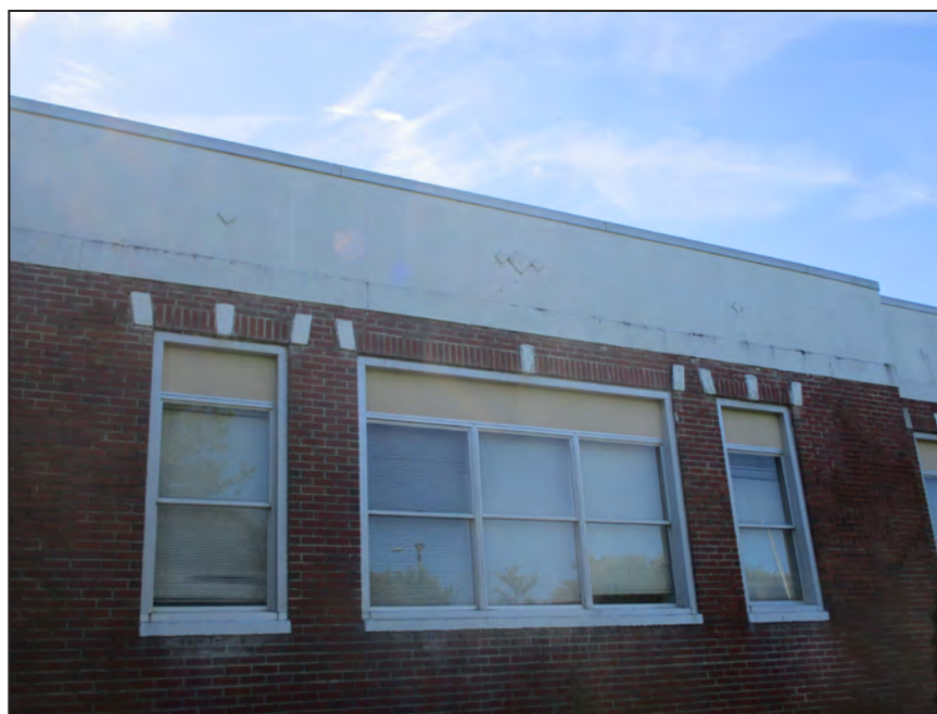
Photograph 2: Detail of window and cornice on Dixon School's Front Hall ; looking east. (2018)
